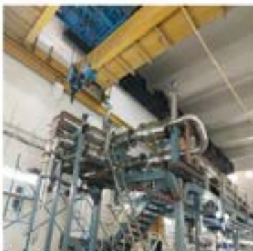
LHE CRYO TRANSFER LINE AT VECC KOLKATA
