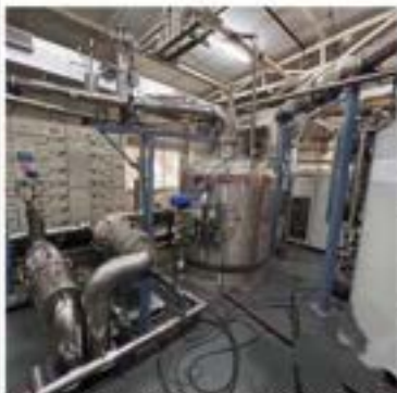
LHE CRYO TRANSFER LINE AT VECC KOLKATA
